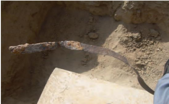
Figure 9. Part of solid zinc galvanized steel tape creating the ring earth electrode around the 220 kV transmission line tower foot after 4 years service in soil.
