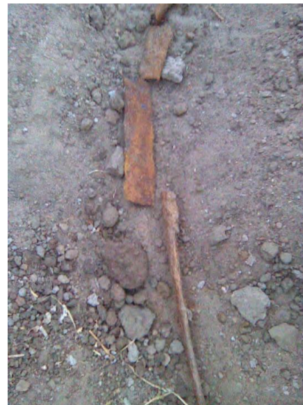
Figure 10. Part of solid zinc galvanized steel tape of the 110 kV transmission line tower earth electrode after 6 years service in soil.
