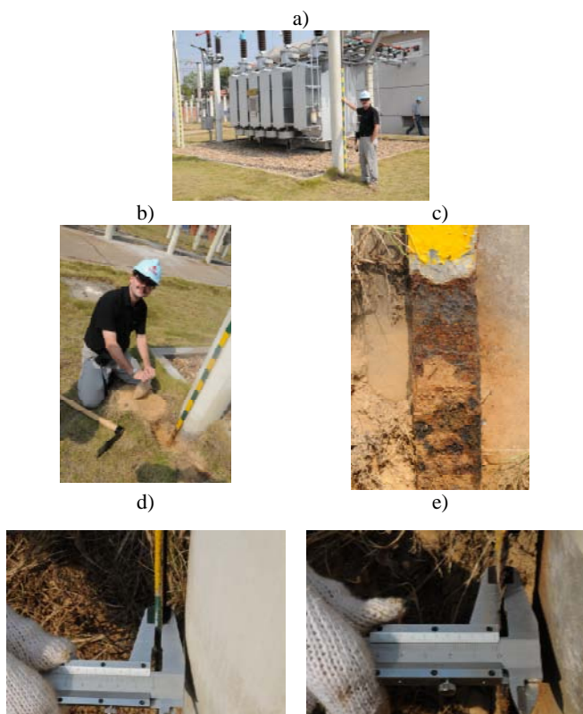
Fig.2. Pictures of 110 kV substation earth electrode inspection with significant corrosion damages after 10 years exposure in soil: a) general view of substation, b) uncovering of soil upper layer, c ÷ d) measurements of earthing tape thickness.
